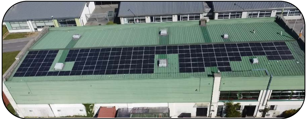
• Solar panels on Dunshaughlin Community Centre's roof.
